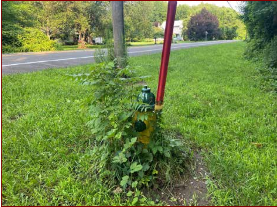
FIRE HYDRANT ON OSWEGO ROAD FRONTAGE
